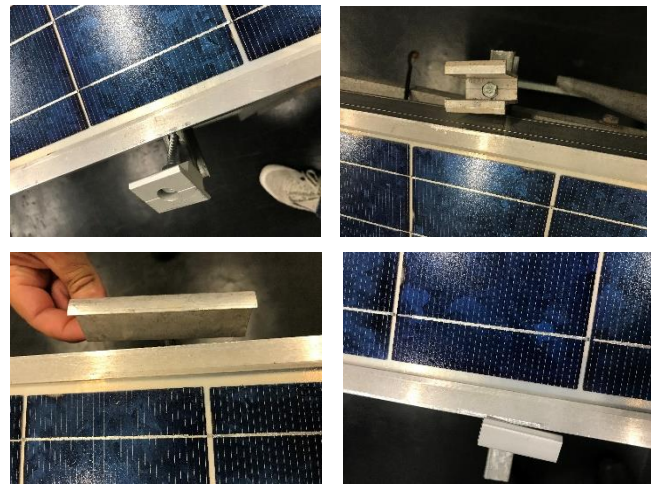
Figure 17 a), b), c) e d): Connectors after current tests.
